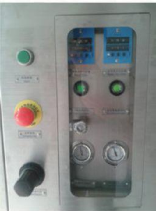
NEW CONTROL PANEL
